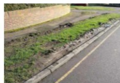
Parking causing damage to the verge
